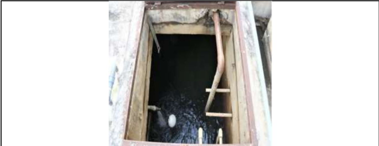
Water tank equipped with automatic float in Faculty of Public Health
