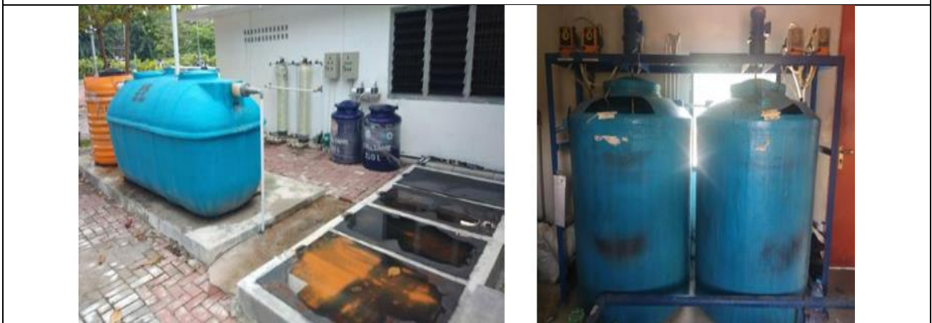
3. Waste Water Treatment Plant for Isolation Room at USU Hospital
